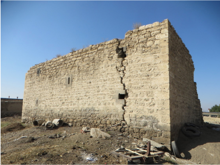
Figure 5 Dirshk S.Sargis cracks in the east wall. 2018. © Boriani M.
