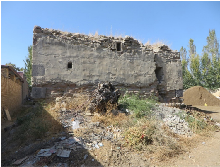
Figure 7 Akhtekhaneh S.Astvatstatsin, erosion of the top caused by the rain and rising damp from the ground © Boriani M.
