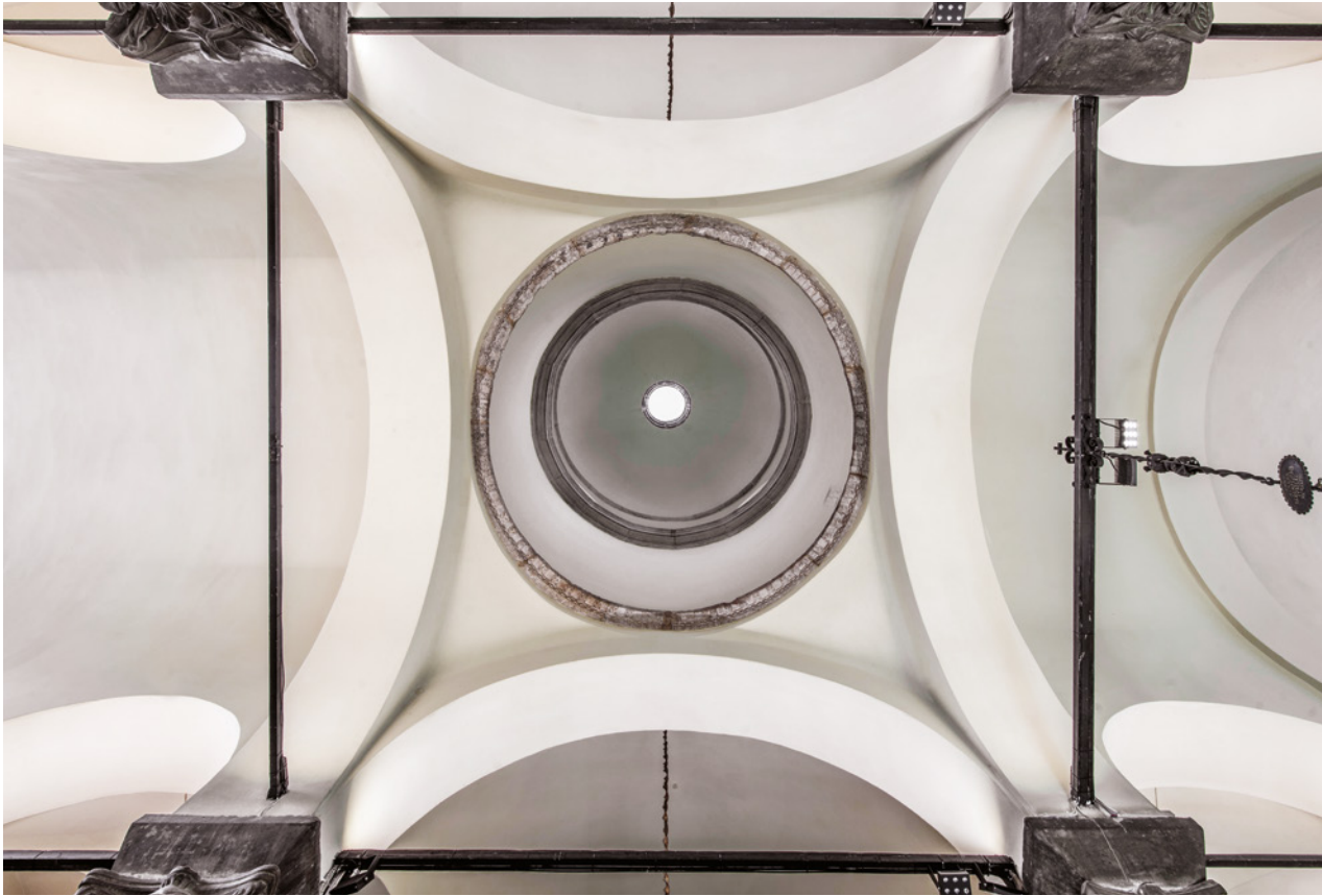
Figure 1 Church of San Giacomo di Rialto, Venice. Network of metal struts supporting columns and arches
