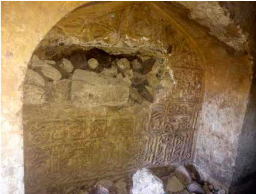
Figure 7. Funerary complex of the Bahmani dynasty. Tombstone in the north-western niche with a large crack in the upper part. Ashtur, India (photo: S. Mondini, 2015)
